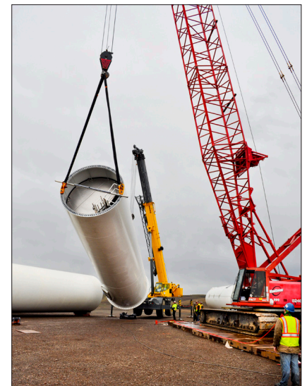
PSE contractors use cranes that extend 390 feet into the air to erect the 149 tall wind-power turbines constructed for Phase I of the Lower Snake River Wind Project in Garfield County.
