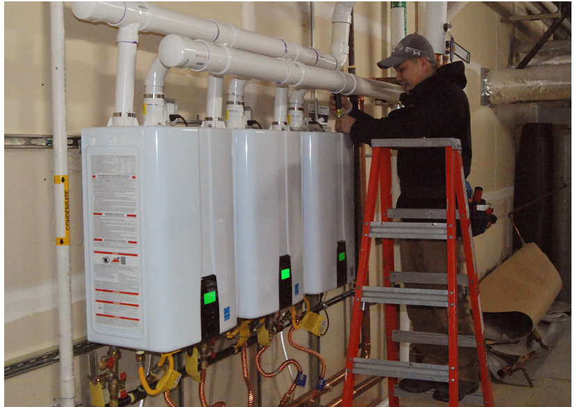
Steilacoom School District replaced failed water heaters with a high-efficiency, on-demand sequenced water-heating system that ties into the building’s automation system.
